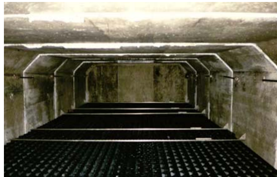
Minocqua, WI, MCTT main settling chamber
