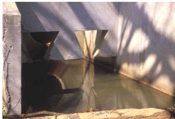
Slot energy dissipators at pond outlet
