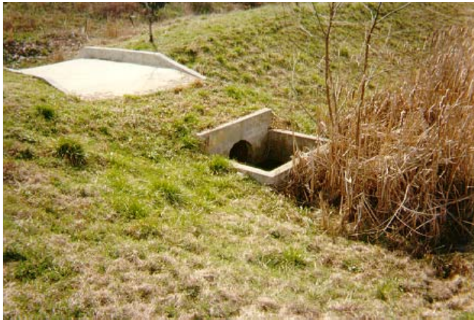
Birmingham, AL pond outlet structure, showing cattails partially blocking 22 in orifices through concrete wall (John Easton photo)
