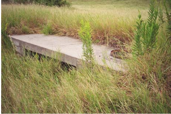
Box outlet emergency spillway at Gulf Port, MS, pond
