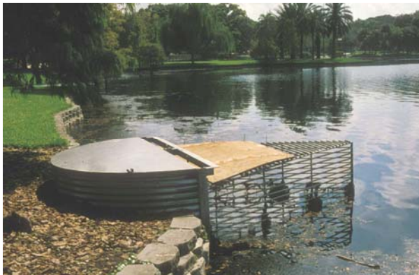
Trash fence at pond inlet at Orlando pond, FL
