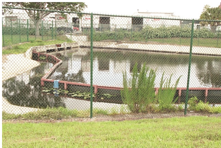
Orlando, FL, settling ponds to remove floc after alum injection, before discharge to lake
