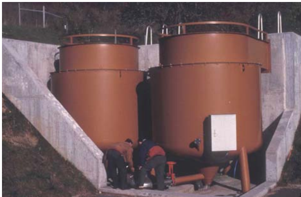
Gravity separation of wet weather solids in CSO swirl concentrators at Tangen, Germany
