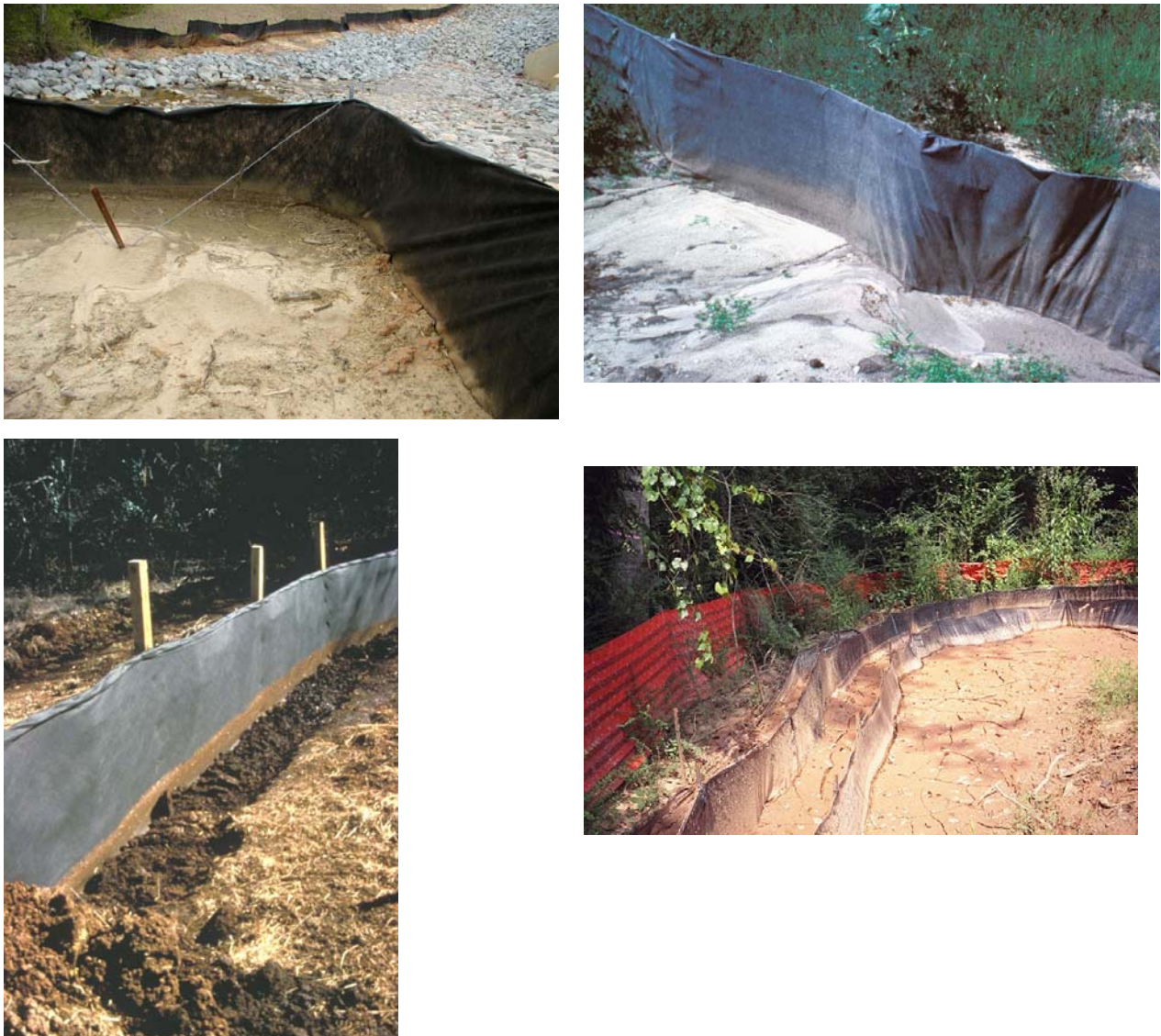
Figure 138. Filter fence installations showing areas of sedimentation where water pools behind the fences
