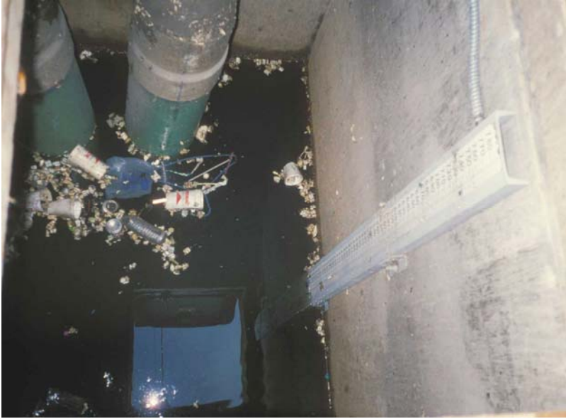
Figure 22. Oil and grease trap before downtown detention pond in Austin, TX.
