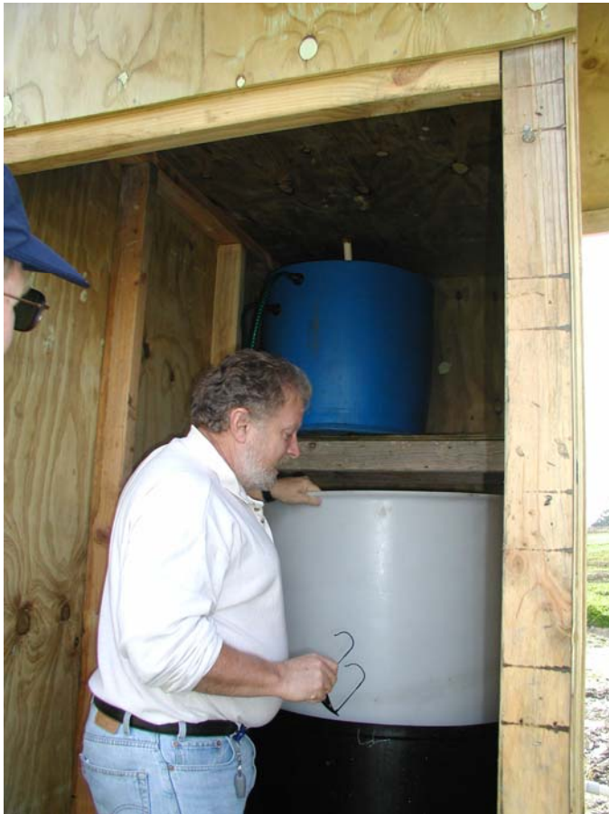
Figure 20. Main components of Auckland Regional Council rainfall-driven chemical dosing system.
