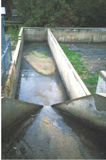
Sedimentation forebay before vertical flow sand filter at Austin, TX
