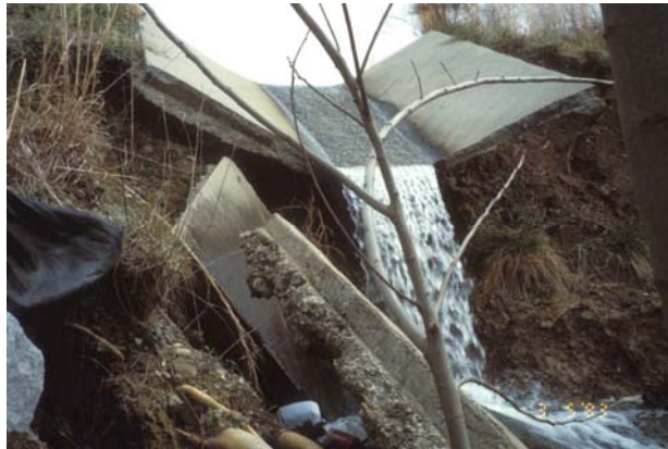
Broken concrete spillway due to undercutting (photo by Mark Burford)
