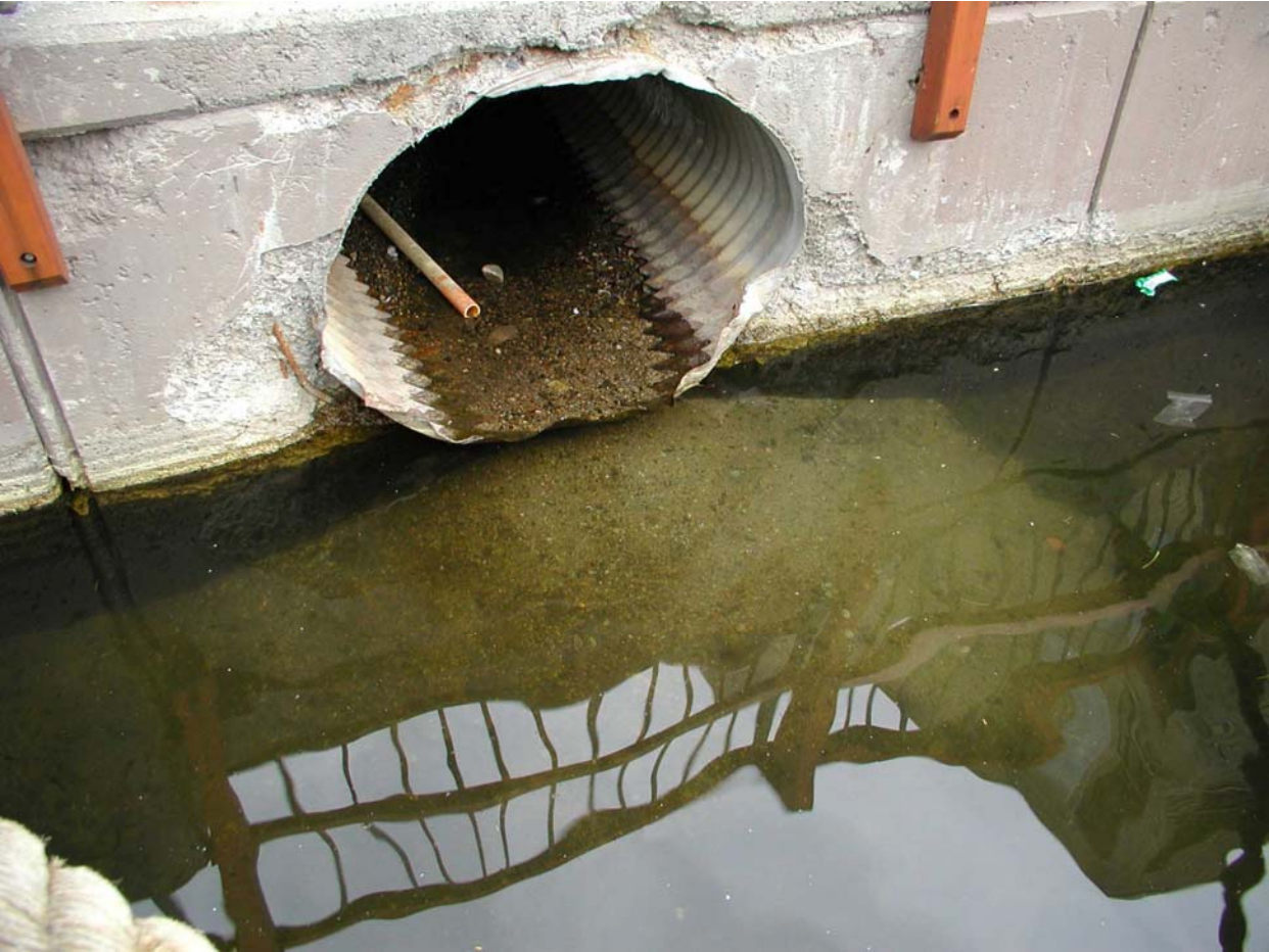
Figure 65. Bedload sediment accumulation in sewerage and near outlet in pond (Snowmass, CO).
