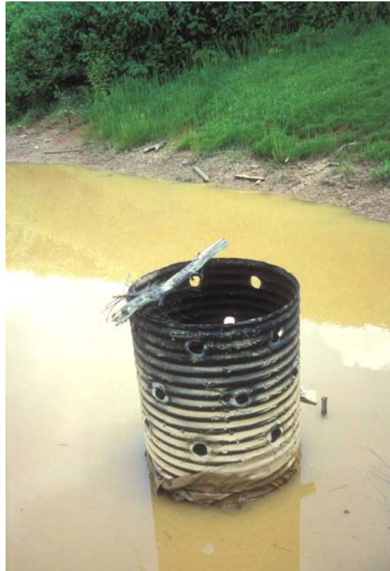
Typical perforated riser vertical stand-pipe at temporary pond, with no bar screens
