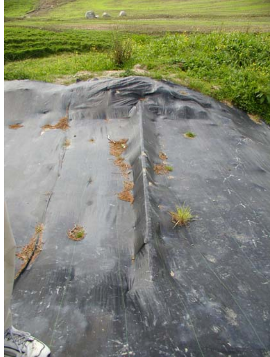
Temporary outlet control at construction site pond using a plastic membrane over a timber weir, Auckland, NZ
