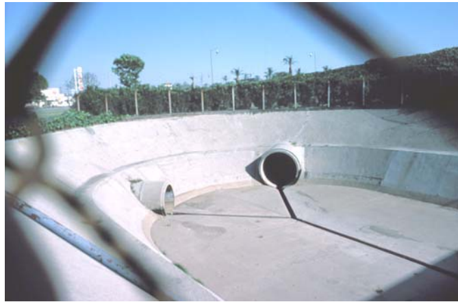
Los Angeles River, CA, stormwater pumping station forebay
