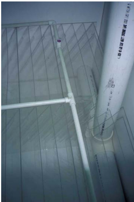
Lamella plates and aerator distributors at pilot-scale MCTT, Birmingham, AL
