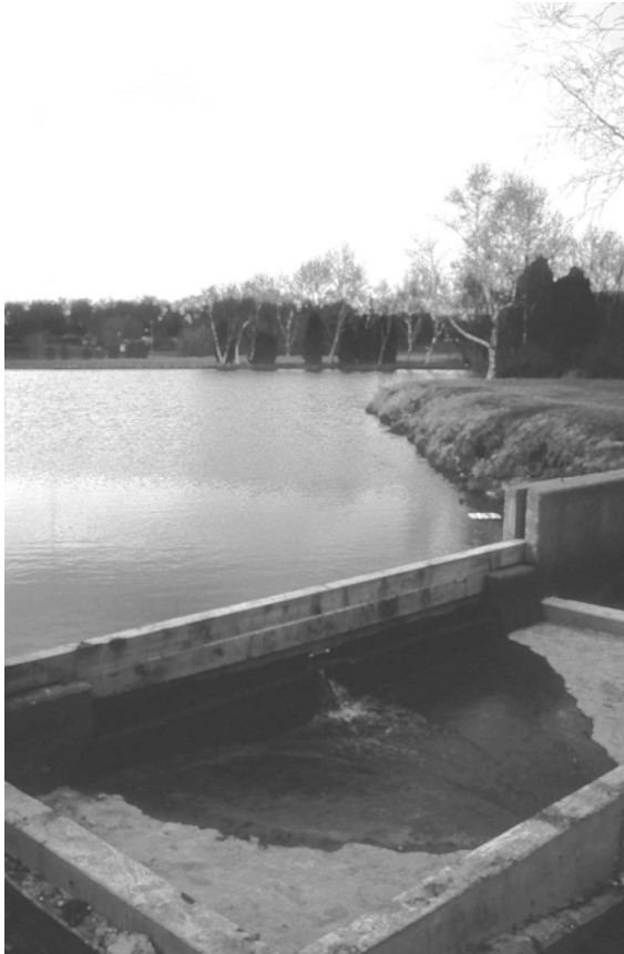
Adjustable spillway using boards in grooved weir Figure 40. Outlet structures at wet detention ponds.
