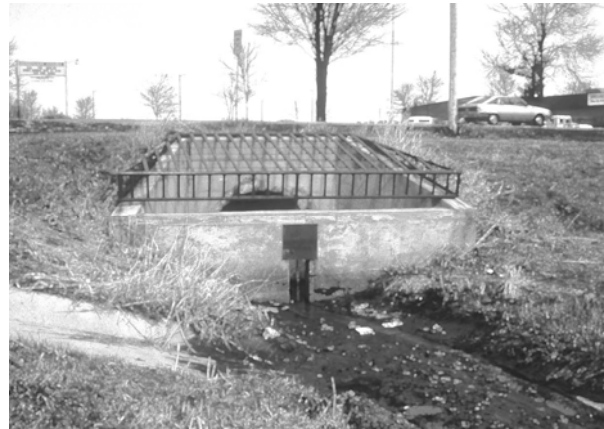
Safety bars over pond outlet
