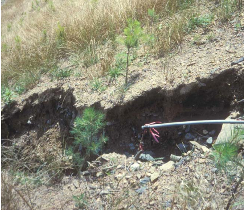
Figure 28. Slope erosion due to seepage through pond dam.
