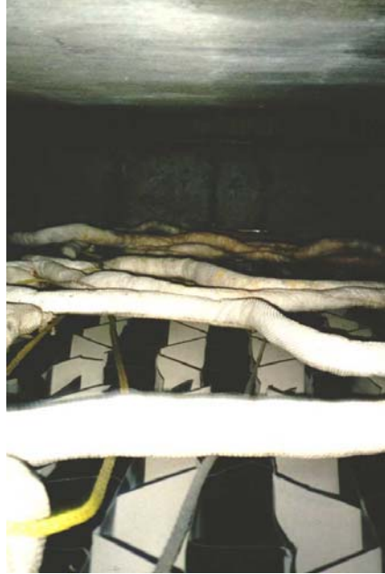
Inclined tube settlers and sorbent socks at MCTT installation in Milwaukee, WI
