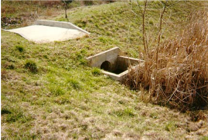
Figure 115. Outlet structure, showing cattails partially blocking the 22 in orifices through concrete wall.
