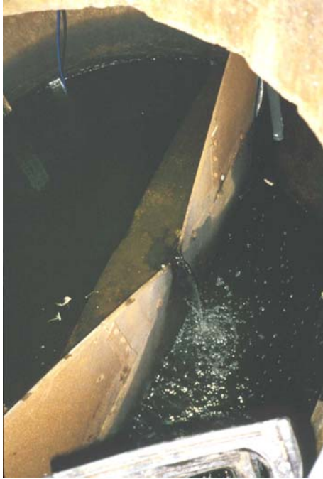
Retro-fitted v-notch weir in place of large rectangular weir at Monroe St. pond in Madison, WI
