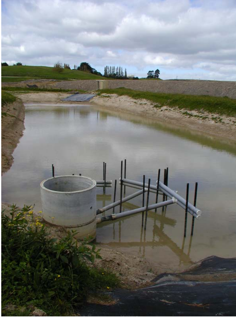
Figure 21. Multi-level, perforated, floating discharges (decants) to better retain floc.
