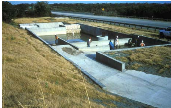
Austin, TX, MoPac Highway treatment unit using accident discharge diversion capture pond, dry pond, and horizontal flow sand filter
