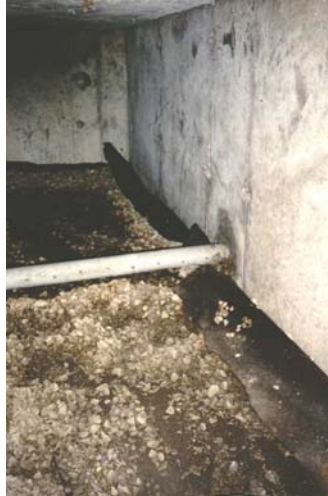
Ruby Garage, Milwaukee, WI, MCTT filtration/sorption chamber
