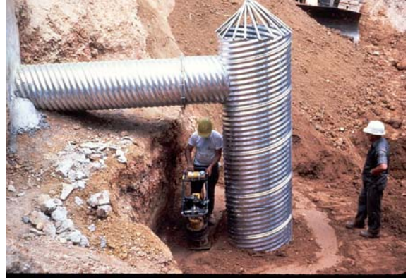
Vertical riser with safety bars, but culvert outlet should normally be placed near pond bottom to allow drainage for maintenance (State of Maryland photo)
