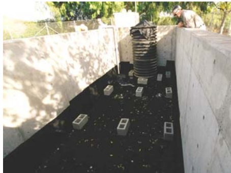
Via Verde Park and Ride, Caltrans, Los Angeles, CA, MCTT filtration/sorption chamber
