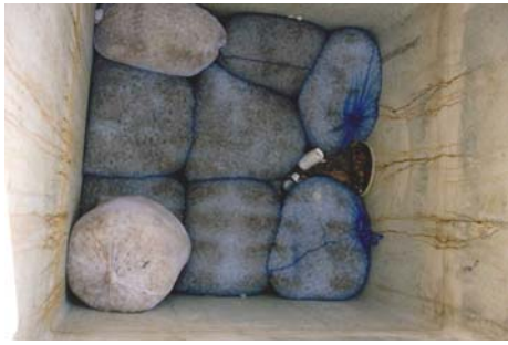
Lakewood Park and Ride, Caltrans, Los Angeles, CA, MCTT inlet chamber
