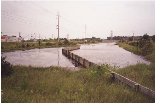
Baffle fence constructed in pond to separate inlet (to right) from pond outlet (to left), forcing water to travel further down pond length.
