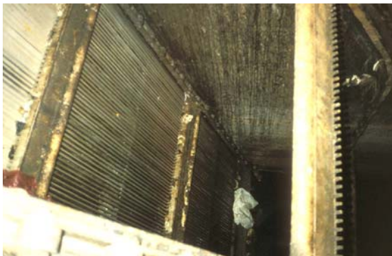
Bar screen at Boston CSO facility for trash control
