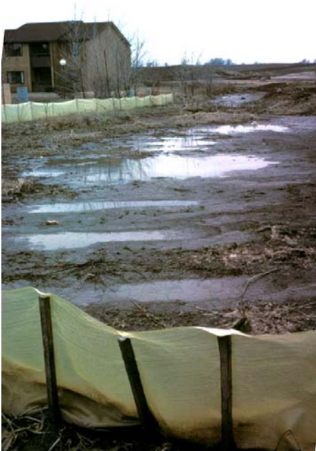
Middleton, WI, pond (heavy erosion filled pond)
