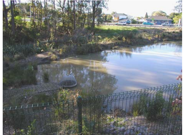
Debris dome over Auckland, NZ, pond riser outlet
